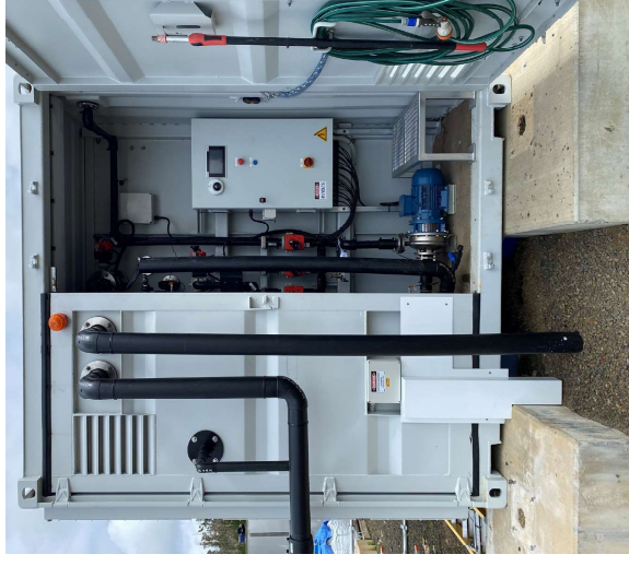
EnPhytoBox plant room and remote operation system
